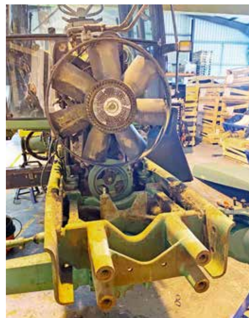
A Flexxair reversible cooling fan will be fitted in place of the viscous coupled original. The latter and the entire cooling system was found to be in good order, although the coolant drained from the system had clearly not been changed in many years.
